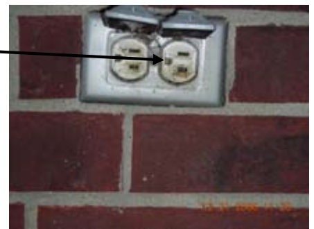
Exterior out near A/C missing weathertight cover
