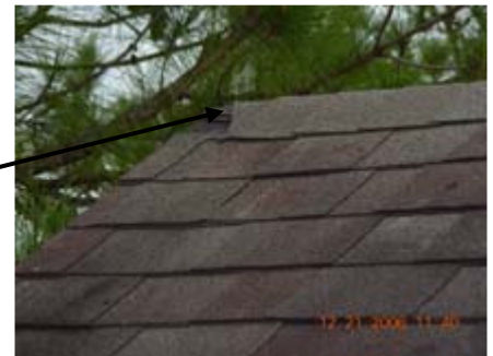
Torn shingle on roof ridge
