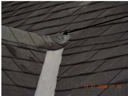
Roof ridge needing tar
